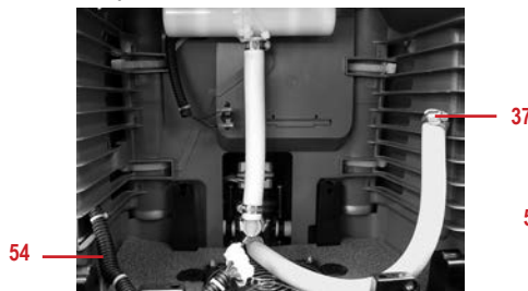
Compressor Box - Serial # "N"
